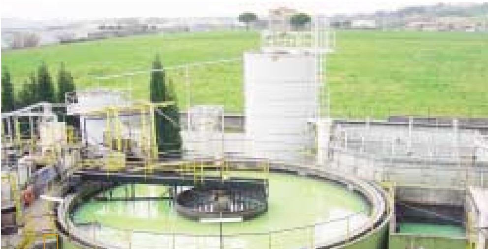
Waste water treatment station at the cathode-ray tube production site at Anagni.
