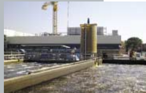
Industrial effluents treatment station at Technicolor laboratory in Rome.
