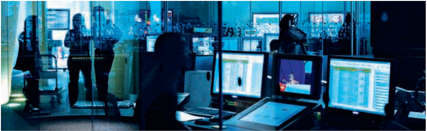
Thomson manages play-out facilities for TV Channels and out-of-home networks from facilities in Paris, London, Atlanta, San Francisco and Tokyo
